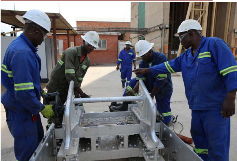
Skip assembly at the shaft (installation of cluster frames on the bridge)
